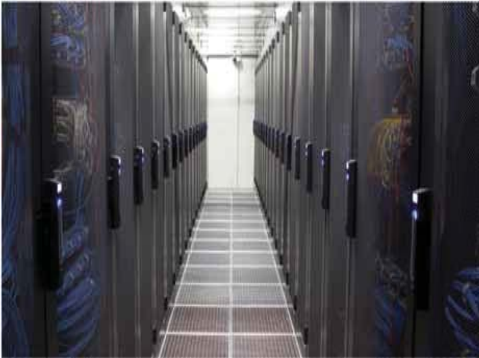
@Lock Solution: MLR handles in a colocation datacenter
